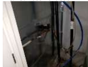
Pic. 47: Water main
