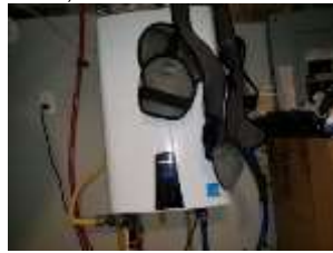
Pic. 50: Tankless hot water system
