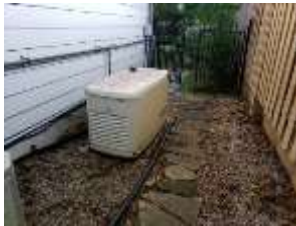
Pic. 9: Backup gas generator
