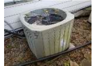
Pic. 8: AC unit
