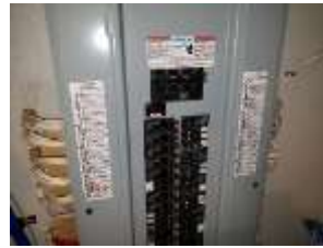
Pic. 51: 200 Amp breaker panel
