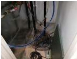
Pic. 46: Sanitary pump – should be sealed to prevent off gassing
