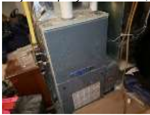
Pic. 49: Gas furnace
