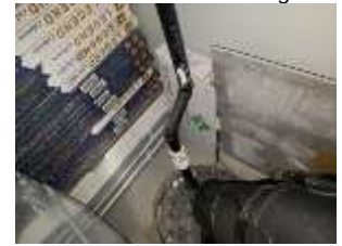
Pic. 52: Sump pump
