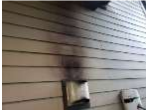
Pic. 5: Family room gas fireplace vent – darkening on the siding recommend having the fireplace reviewed and cleaned
