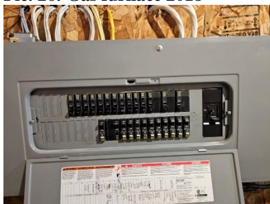
Pic. 29: 200 amp breaker panel
