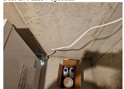
Pic. 30: Outlet and loose wiring should be properly secured in cold room
