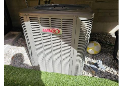
Pic. 3: AC unit 2018
