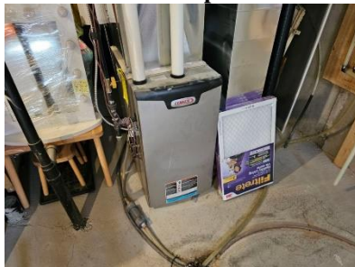
Pic. 26: Gas furnace 2018
