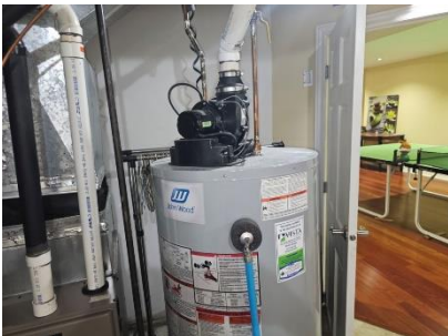
Pic. 28: Hot water tank 2017
