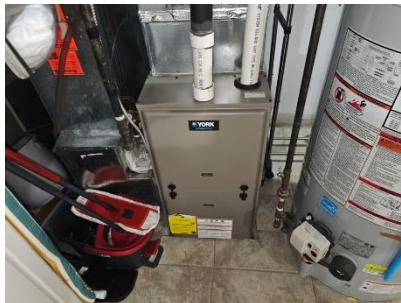
Pic. 29: Gas furnace
