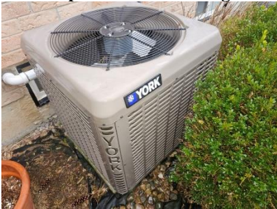
Pic. 7: AC unit 2016
