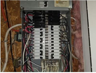
Pic. 31: 100 amp breaker panel
