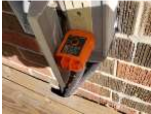
Pic. 5: Exterior GFCI need to be replaced
