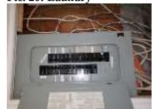
Pic. 24: 100 amp breaker panel
