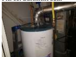
Pic. 22: Water heater 2011
