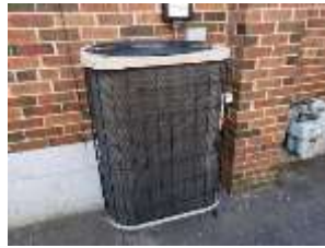
Pic. 2: AC unit 2008
