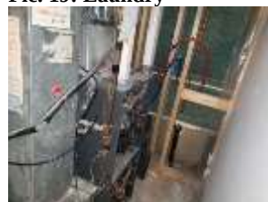
Pic. 23: Gas furnace 2013
