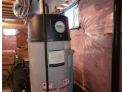
Pic. 32: Rental hot water tank
