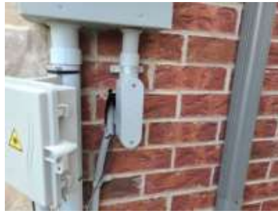
Pic. 2: Gap around main power line should be sealed
