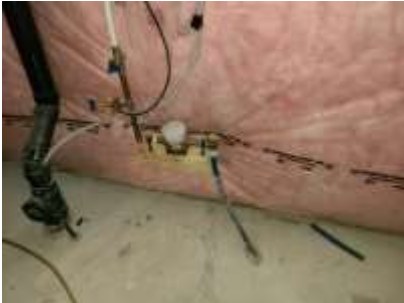
Pic. 31: Water main
