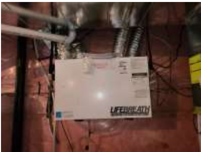
Pic. 34: HRV system
