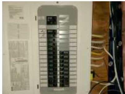
Pic. 35: 100 amp breaker panel
