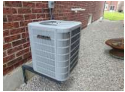
Pic. 3: AC unit
