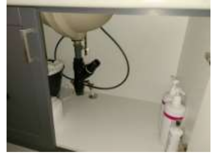
Pic. 15: Left side sink not functional – to be repaired before closing
