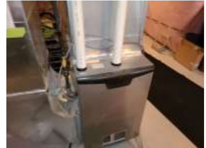
Pic. 33: Gas furnace
