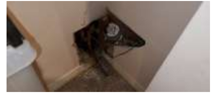
Pic. 30: Water main
