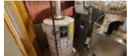
Pic. 27: Retnal hot water tank 2011
