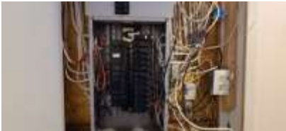
Pic. 31: 100 amp breaker panel
