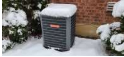
Pic. 2: AC unit 2008
