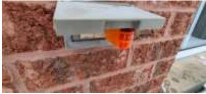
Pic. 4: Rear GFCI won't trip – re[;ace
