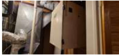
Pic. 29: HRV system
