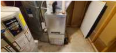
Pic. 28: Gas furnace 2019
