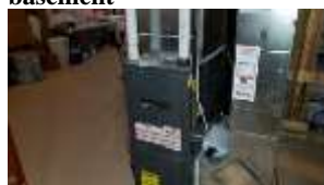
Pic. 30: Gas furnace
