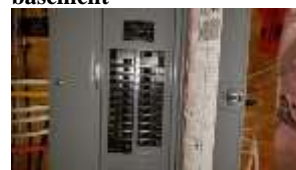
Pic. 31: 100 amp breaker panel
