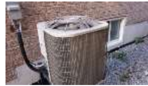
Pic. 3: AC unit
