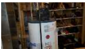
Pic. 29: Rental hot water tank
