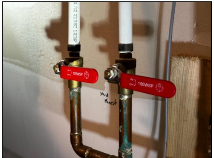
31. Hosebib shut off valves
