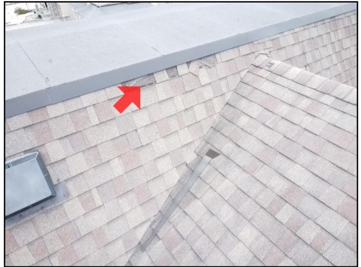
4. Blown away Asphalt Shingles
