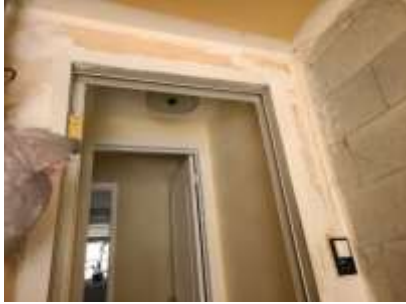
Pic. 4: Auto closer is needed for garage entry door
