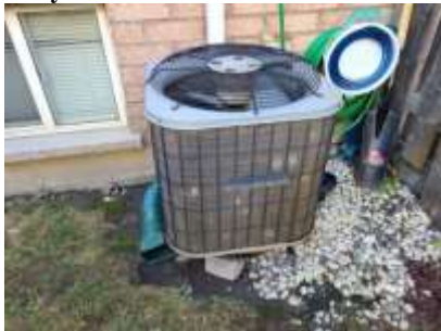
Pic. 7: AC unit 2002
