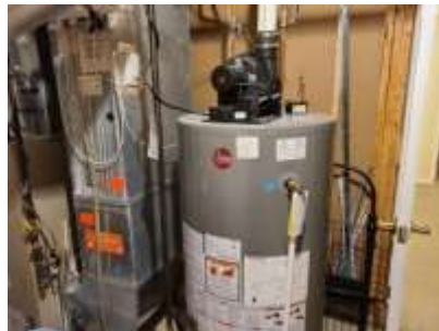
Pic. 26: Rental hot water tank 2016
