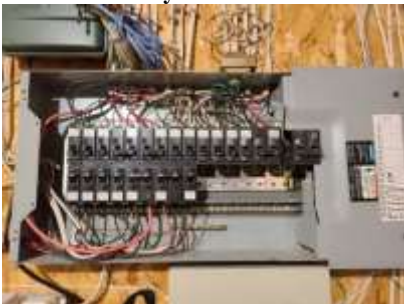
Pic. 28: 100 amp breaker panel
