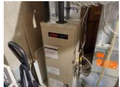
Pic. 27: Original gas furnace 2002
