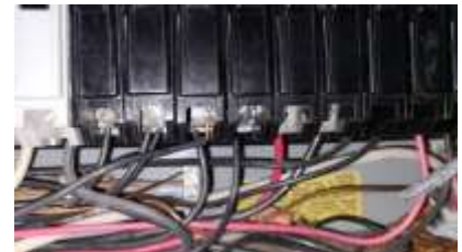
Pic. 30: 2 breakers are double tapped
