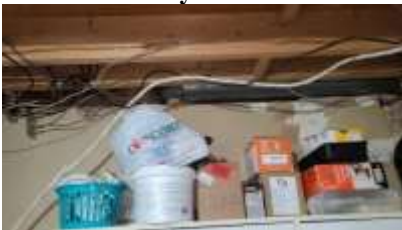
Pic. 28: Loose wires needs to be properly secured
