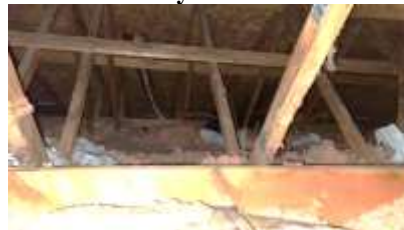
Pic. 8: Attic – Recommend insulation bathroom exhaust vent pipe in the attic
