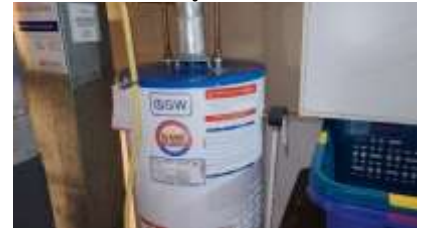
Pic. 27: Hot water tank 2008
