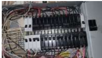
Pic. 29: 100 amp breaker panel
