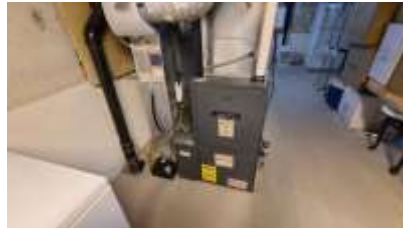
Pic. 26: Gas furnace 2009
