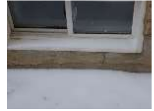
Pic. 4: Typical foundation crack
