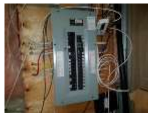
Pic. 43: 100 amp breaker panel – all copper wire
