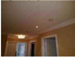
Pic. 25: Smoke & Co detectors outdated
