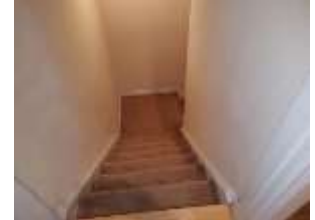
Pic. 36: No handrail upper basement stairs
