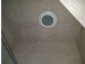
Pic. 22: Shower light not working
