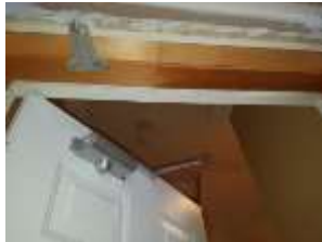
Pic. 10: Auto closer disconnected
