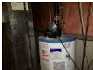
Pic. 42: Rental hot water tank
