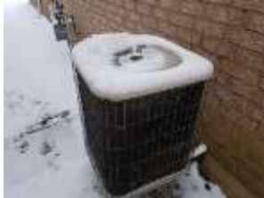
Pic. 5: AC unit 2002
