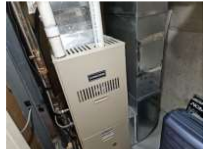
Pic. 24: Gas furnace 2010
