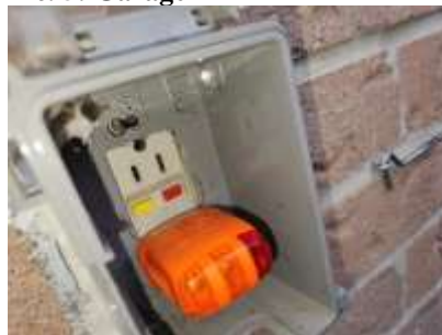
Pic. 8: Rear GFCI outlet will not trip – replace
