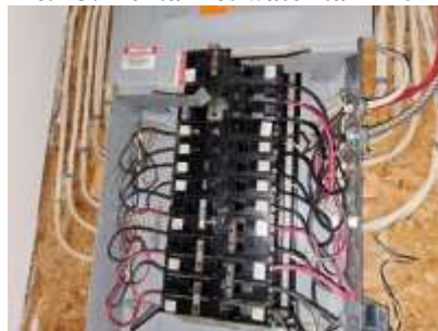
Pic. 26: 100 amp breaker panel
