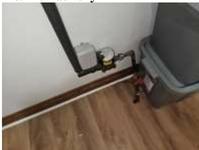
Pic. 25: Water main
