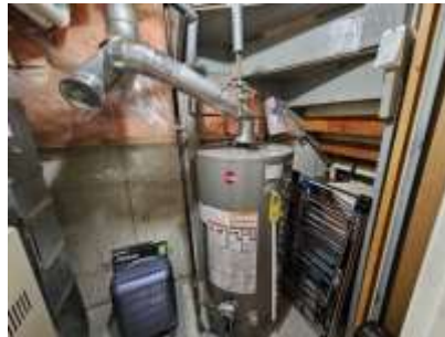
Pic. 23: Rental hot water tank 2022
