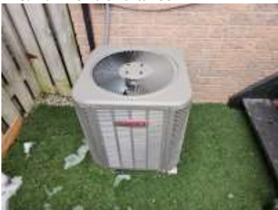
Pic. 7: AC unit 2021
