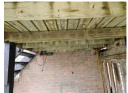
Pic. 9: Recommend review of deck structure
