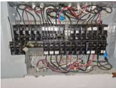
Pic. 7: 100 amp breaker panel
