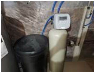
Pic. 29: Water softener
