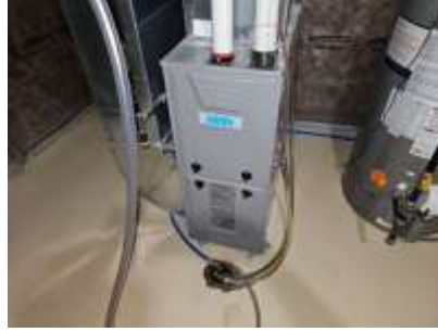
Pic. 32: Gas furnace 2015
