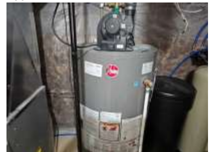
Pic. 30: Rental hot water tank 2015
