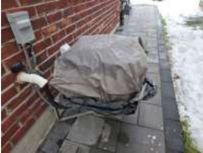
Pic. 4: AC unit 2015
