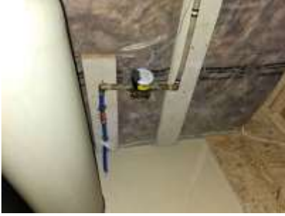
Pic. 31: Water main
