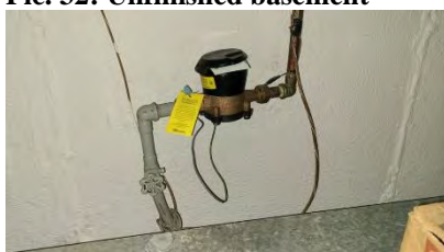
Pic. 35: Water main
