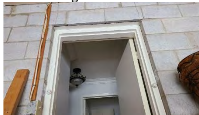
Pic. 11: An auto closer is needed for the garage entry door
