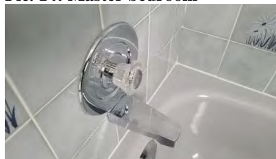
Pic. 17: Tub faucet could not be opened
