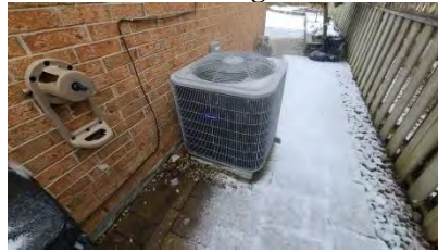
Pic. 5: AC unit 2017
