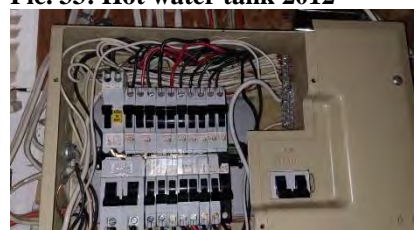
Pic. 36: 100 amp main electrical panel
