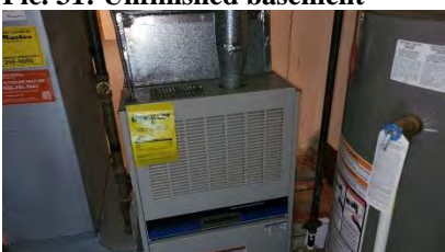
Pic. 34: Gas furnace 2000
