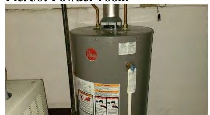
Pic. 33: Hot water tank 2012
