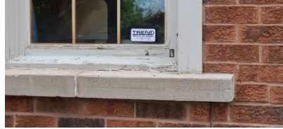
Pic. 5: Window frames are aged condition
