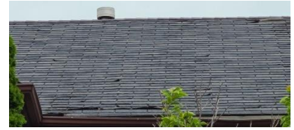
Pic. 3: Aging roof covering
