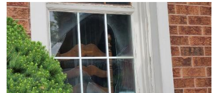
Pic. 15: Broken window panel
