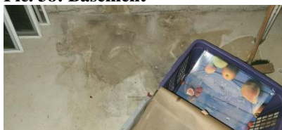
Pic. 41: Signs of past foundation leak, have reviewed and repaired accordingly
