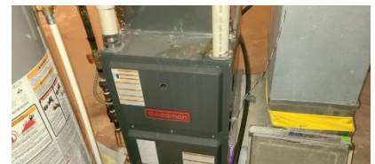
Pic. 45: Gas furnace
