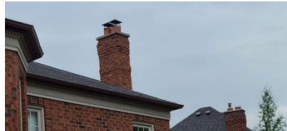
Pic. 8: Chimney, in need of some repairs
