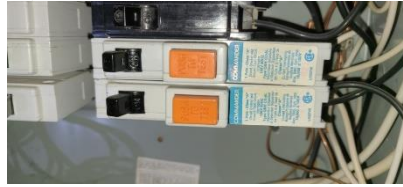
Pic. 47: GFCI breakers wont trip when tested and need to be replaced
