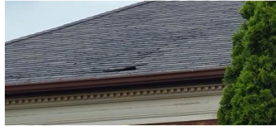
Pic. 2: Aging roof covering
