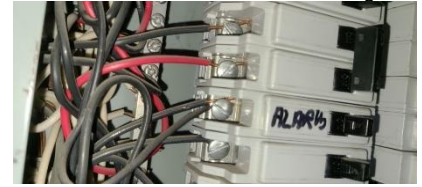
Pic. 48: Double tapped breaker
