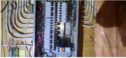
Pic. 46: 200-amp breaker panel
