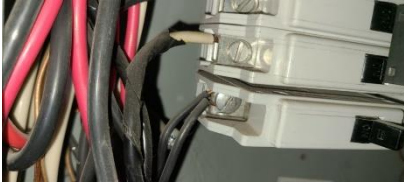
Pic. 49: Double tapped breaker
