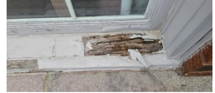
Pic. 6: Some window frames have noticeable rot
