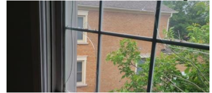
Pic. 24: Broken glass panel
