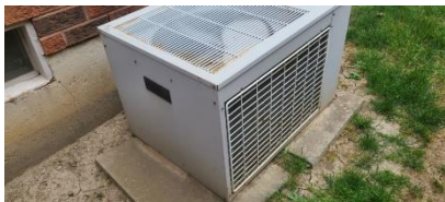
Pic. 10: Aged AC unit, budget for replacement
