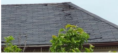
Pic. 4: Aging roof covering
