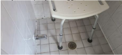
Pic. 22: Regular caulking maintenance needed in shower
