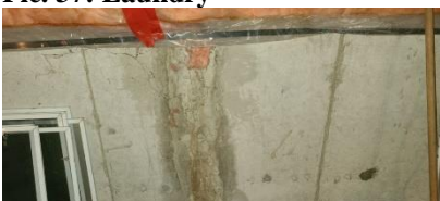
Pic. 40: Signs of past foundation leak, have reviewed and repaired accordingly
