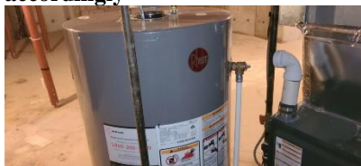
Pic. 44: Rental hot water tank
