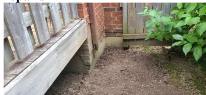
Pic. 11: Downspout extension needed
