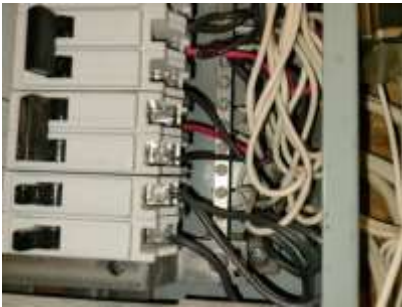
Pic. 37: Couple of breakers double tapped
