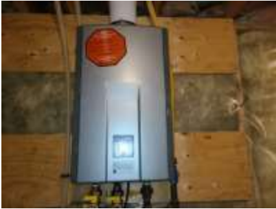
Pic. 34: Tankless hot water system
