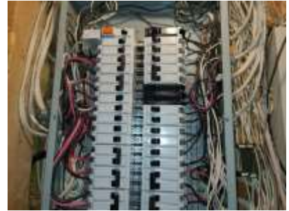
Pic. 36: 200 amp breaker panel with all copper wire
