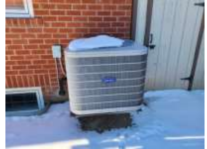
Pic. 6: AC unit 2008
