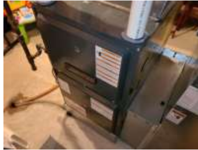
Pic. 35: Gas furnace 2019
