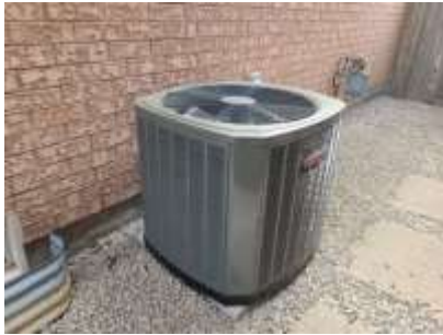
Pic. 4: AC unit 2013
