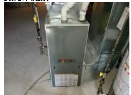
Pic. 30: Gas furnace 2014
