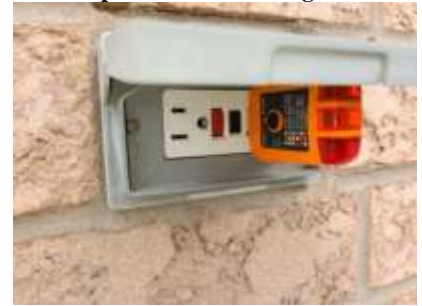
Pic. 6: Exterior GFCI outlet needs to be replaced
