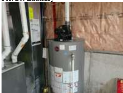
Pic. 29: Rental hot water tank 2016
