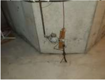
Pic. 31: Water main
