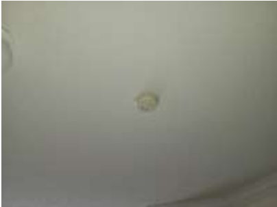
Pic. 19: Smoke detectors are dated and needs to be replaced
