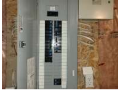
Pic. 32: 200 amp breaker panel
