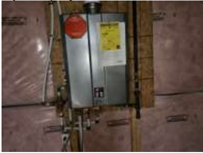
Pic. 31: Tankless hot water system 2010
