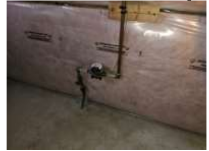
Pic. 33: Water main
