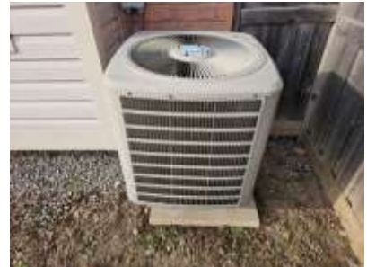
Pic. 9: AC compressor 2012
