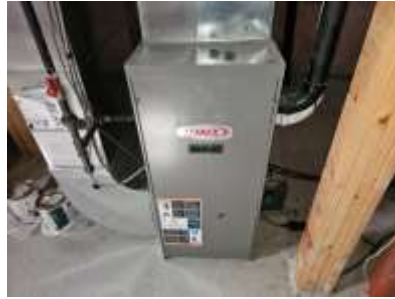
Pic. 32: Gas furnace 2011
