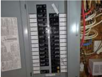
Pic. 34: 100 amp breaker panel
