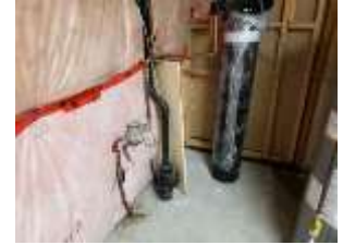
Pic. 32: Water main and softener
