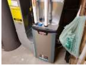
Pic. 30: Gas furnace 2018
