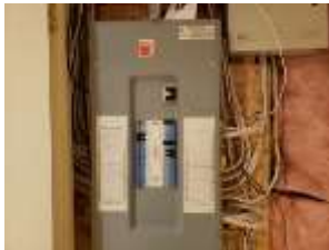
Pic. 33: 100 amp breaker panel
