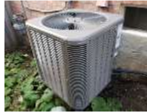
Pic. 3: AC unit 2018
