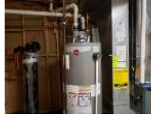
Pic. 31: Rental hot water tank 2018
