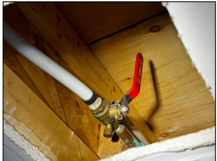
23. Hosebib shut off valve
