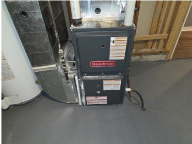
Pic. 34: Gas furnace 2022
