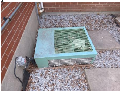
Pic. 7: Old AC compressor – budget for replacement
