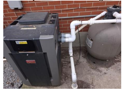
Pic. 6: Pool pump and heater
