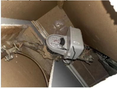
Pic. 31: Water main
