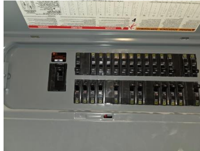
Pic. 35: 100amp breaker panel
