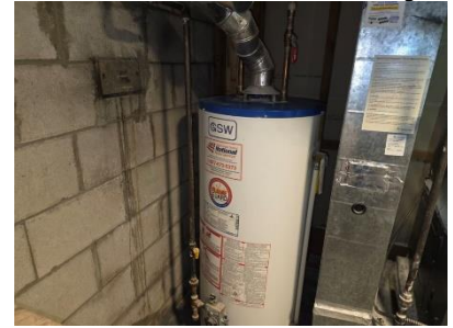
Pic. 33: Rental hot water tank 2008
