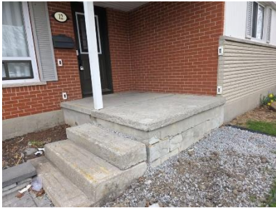
Pic. 4: Railing needed on front porch
