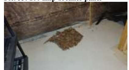
Pic. 36: Insulation needs to be replaced
