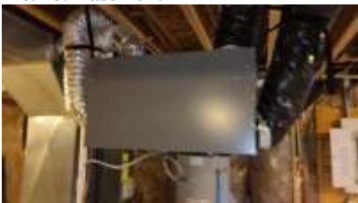
Pic. 31: HRV system
