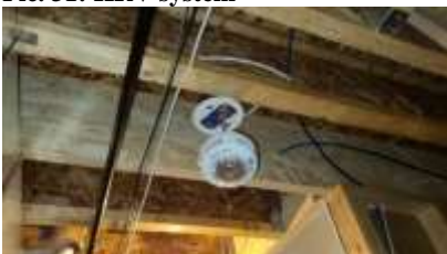
Pic. 34: Smoke detector needs to be reconnected
