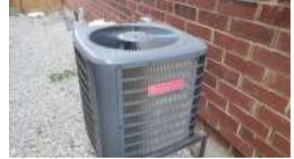
Pic. 3: AC unit 2016
