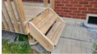
Pic. 5: Deck stairs need repair
