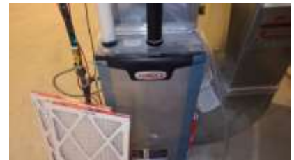
Pic. 30: Gas furnace 2016
