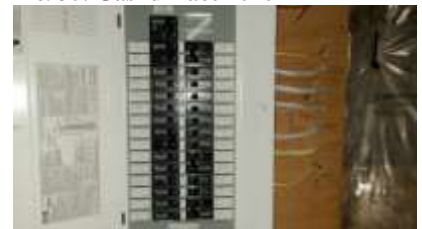
Pic. 33: 100 amp breaker panel
