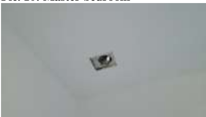
Pic. 13: Missing cover for exhaust fan
