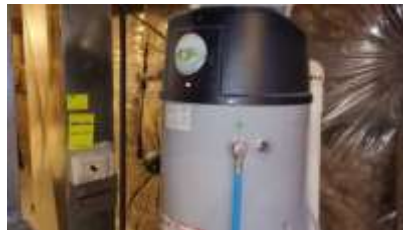
Pic. 29: Rental hot water tank
