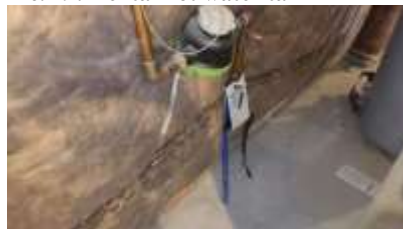
Pic. 32: Water main
