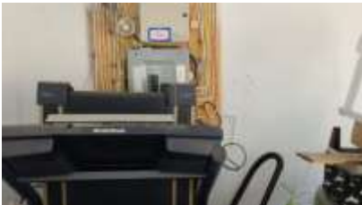
Pic. 25: 100 amp breaker panel
