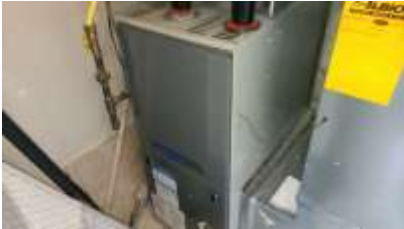
Pic. 22: Gas furnace 2007
