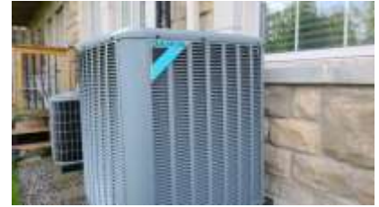
Pic. 3: AC unit 2017
