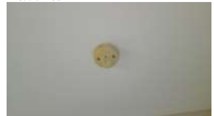
Pic. 12: Smoke / CO detectors dated on 2 nd floor
