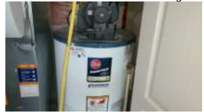
Pic. 21: Rental hot water tank 2006
