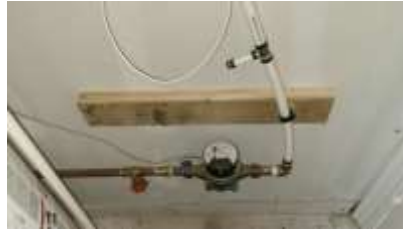
Pic. 23: Water main
