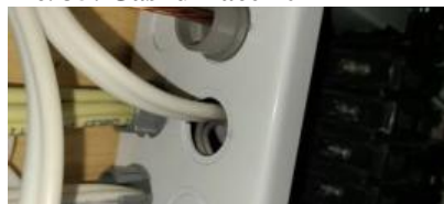
Pic. 38: Grommet needed for wire entering panel
