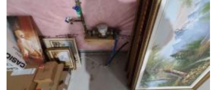
Pic. 33: Water main
