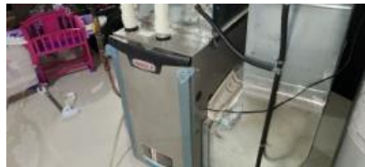
Pic. 35: Gas furnace 2017
