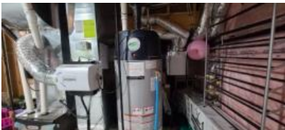
Pic. 34: Rental hot water tank 2017
