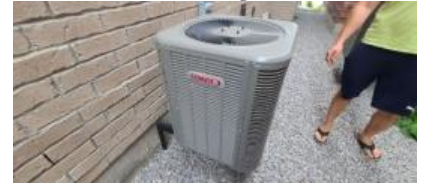
Pic. 6: AC unit 2019
