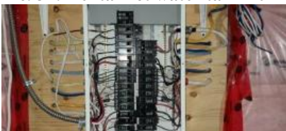
Pic. 37: 100 amp breaker panel
