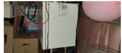
Pic. 36: HRV system
