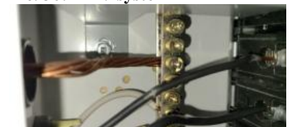
Pic. 39: Wire appears to be nicked, have check and corrected as necessary
