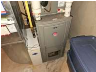
Pic. 41: Gas furnace 2021
