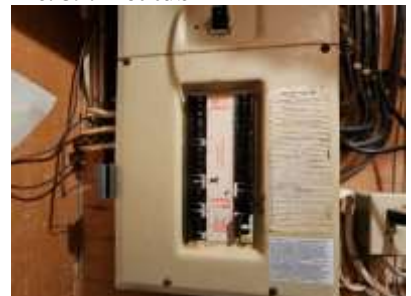
Pic. 42: 200 amp breaker panel
