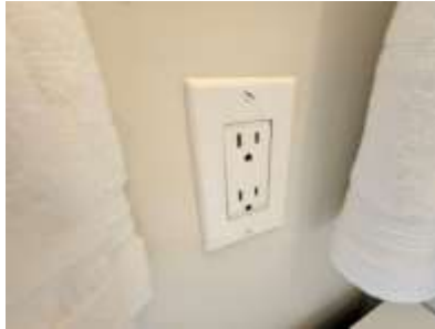
Pic. 17: Outlet should be upgraded to a GFCI protected outlet
