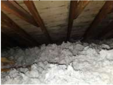
Pic. 13: Some minor staining and possible minor mould growth
