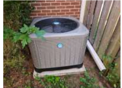
Pic. 9: AC unit 2021
