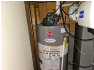
Pic. 40: Rental hot water tank 2023
