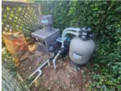
Pic. 8: Pool heater, filter and pump
