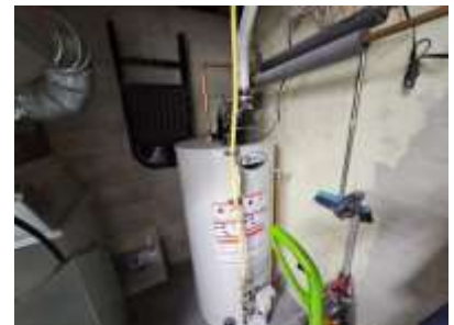
Pic. 30: Hot water tank
