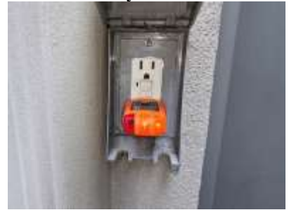
Pic. 6: Rear GFCI outlet trip
