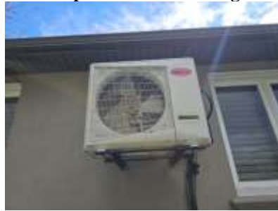
Pic. 5: AC unit
