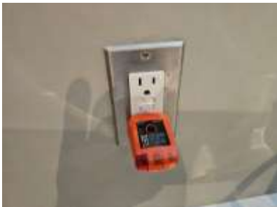
Pic. 25: Left side counter plug has no power
