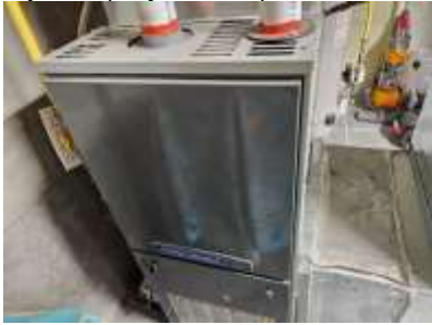
Pic. 31: Gas furnace
