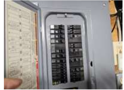
Pic. 33: Breaker panel
