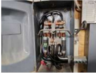
Pic. 32: 100 amp main disconnect
