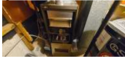
Pic. 26: Original gas furnace 1978
