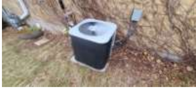
Pic. 4: AC unit 2018
