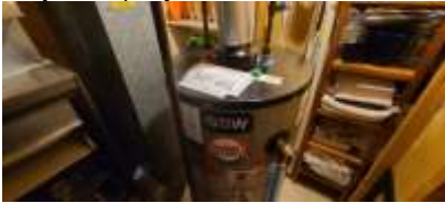
Pic. 25: Rental hot water tank 2015
