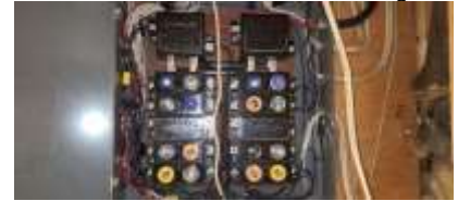
Pic. 27: 100 amp fuse panel – See Electrical Comments
