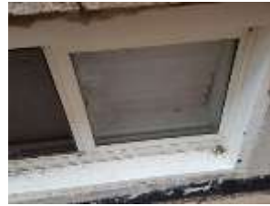
Pic. 7: Cracked basement window
