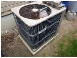
Pic. 5: Original AC unit
