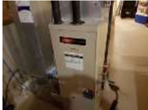
Pic. 26: Original gas furnace
