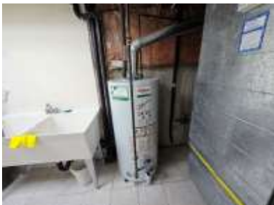
Pic. 28: Rental hot water tank 2012
