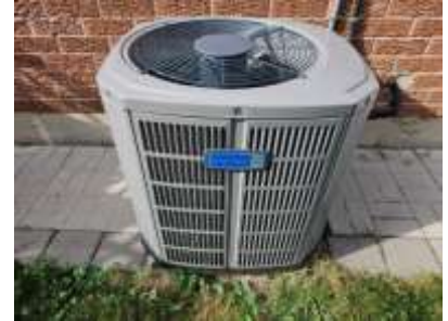
Pic. 6: AC compressor 2022
