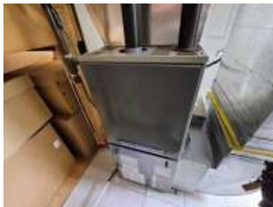
Pic. 29: Gas furnace 2005
