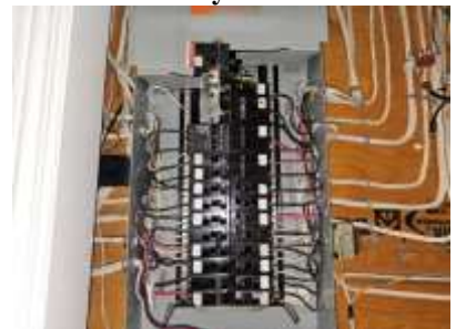
Pic. 30: 100 amp breaker panel
