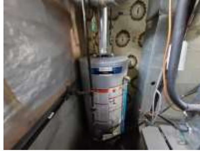
Pic. 32: Water heater 2020
