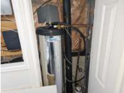
Pic. 34: Water softener
