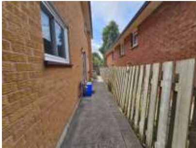
Pic. 7: Fence needs repairs
