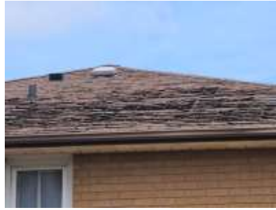
Pic. 2: Roof at the end of its life
