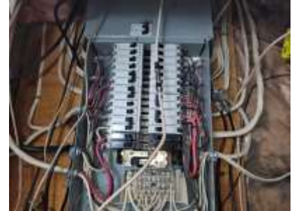
Pic. 36: 100 amp breaker panel
