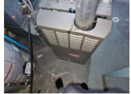
Pic. 33: Gas furnace 2005
