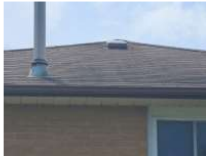
Pic. 5: Rear roof covering – aged
