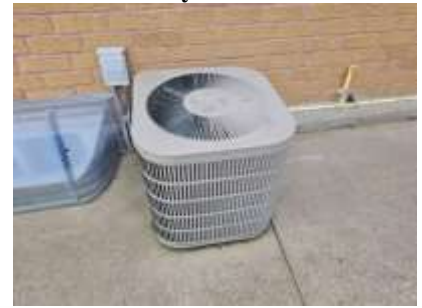
Pic. 6: AC unit 2005
