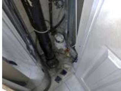
Pic. 35: Water main
