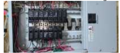
Pic. 24: 100 amp breaker panel
