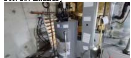
Pic. 21: Rental hot water tank 2015
