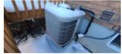
Pic. 3: AC unit 2016
