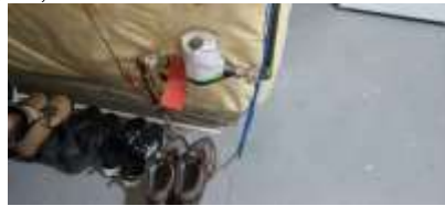
Pic. 23: Water main
