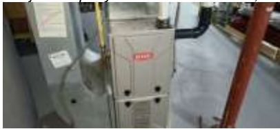
Pic. 22: Gas furnace 2018
