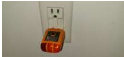
Pic. 8: GFCI outlet not operating as designed and needs to be replaced
