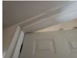
Pic. 7: Auto closer required for garage entry door
