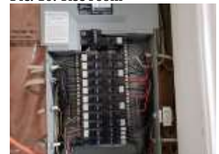
Pic. 20: 100 amp breaker panel
