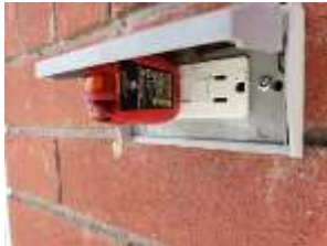
Pic. 5: Rear GFCI outlet needs replacement
