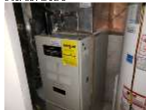
Pic. 19: Original gas furnace
