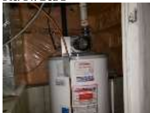
Pic. 18: Rental hot water tank
