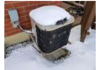
Pic. 4: Original AC unit
