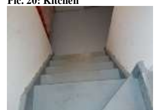
Pic. 24: Basement stairwell requires and handrailing
