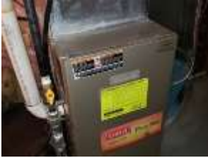
Pic. 29: Original gas furnace
