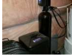
Pic. 31: Water softener
