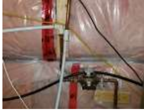
Pic. 30: Water main
