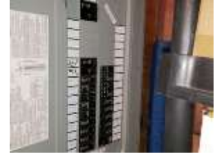
Pic. 32: 100 amp breaker panel
