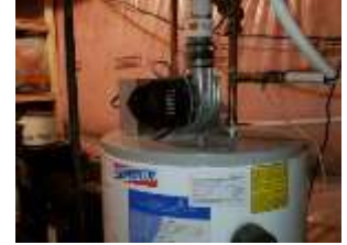
Pic. 28: Rental hot water tank
