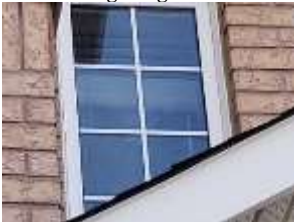
Pic. 33: Bed 3 front window has a cracked glass panel
