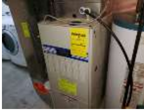
Pic. 29: Original gas furnace
