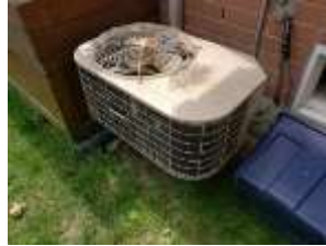
Pic. 6: Original AC unit
