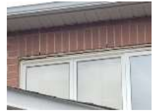
Pic. 4: Caulking maintenance needed around the windows
