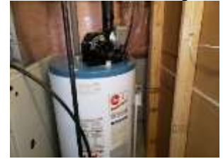
Pic. 28: Rental hot water tank
