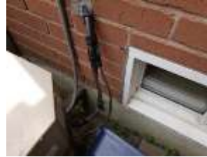
Pic. 7: Insulation missing on refrigerate lines for AC
