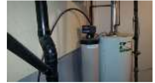
Pic. 52: Water softener
