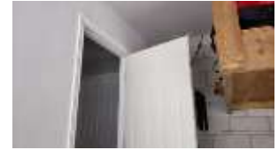
Pic. 32: Auto closer needed for garage entry door
