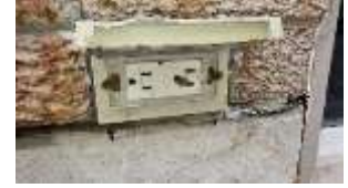
Pic. 4: No power at side exterior outlet
