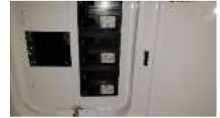
Pic. 56: Openings in panel on the left need to be sealed
