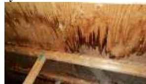
Pic. 19: Old water marks in attic
