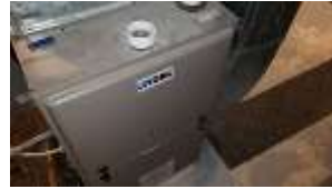
Pic. 51: Gas furnace 2009
