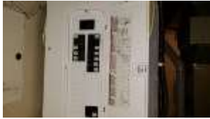
Pic. 53: Sub panel
