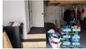
Pic. 31: Railing needed for landing
