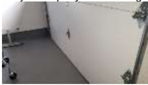
Pic. 33: Safety sensors not aligned
