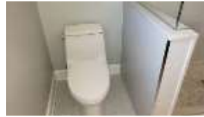
Pic. 27: 2 nd floor bath
