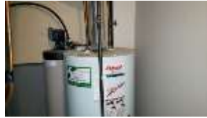
Pic. 50: Hot water tank
