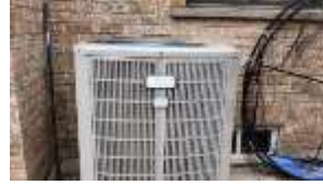
Pic. 3: AC unit 2009
