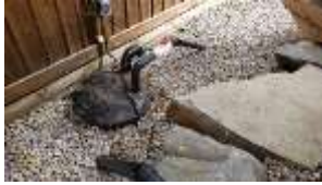
Pic. 13: Sanitary pump
