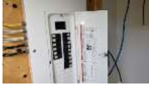
Pic. 14: Sub panel
