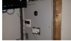
Pic. 15: Cabana hot water system
