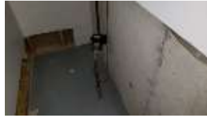
Pic. 54: Water main
