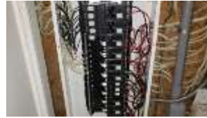
Pic. 55: 200 amp main breaker panel
