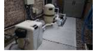
Pic. 16: Pool heater and pumps
