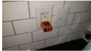
Pic. 42: GFCI no power won't reset
