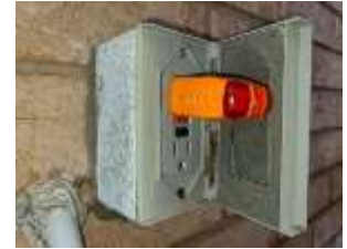
Pic. 4: Front GFCI outlet won't trip
