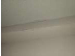
Pic. 26: Old water marks on ceiling – no active moisture
