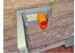
Pic. 8: Rear GFCI outlet won't trip
