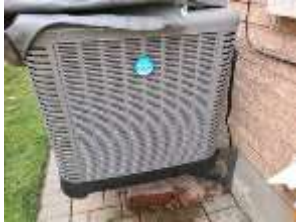
Pic. 5: AC unit 2017
