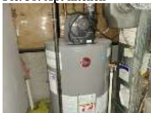
Pic. 42: Hot water tank
