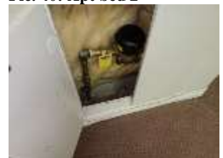
Pic. 44: Water main
