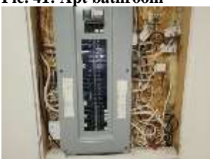
Pic. 45: 200 amp breaker panel with all copper wire
