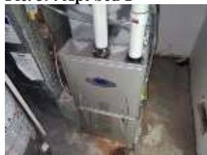
Pic. 43: Gas furnace 2018
