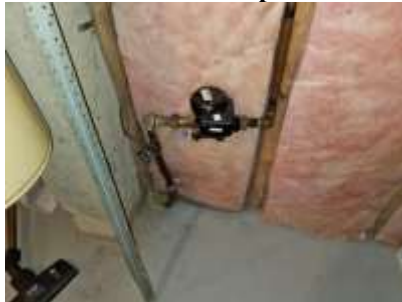
Pic. 38: Water main
