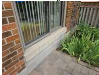
Pic. 8: Steps, railing or patio door needs to be made inoperable for safety
