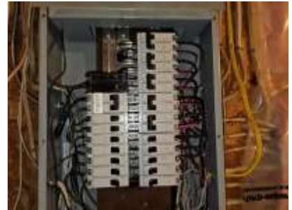
Pic. 39: 150 amp breaker panel
