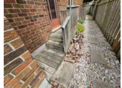
Pic. 6: Side steps in need of repair
