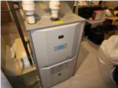
Pic. 37: Gas furnace 2009
