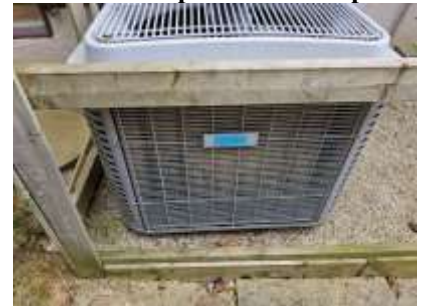
Pic. 9: Ac unit 2009
