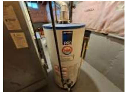
Pic. 36: Hot water tank 2009
