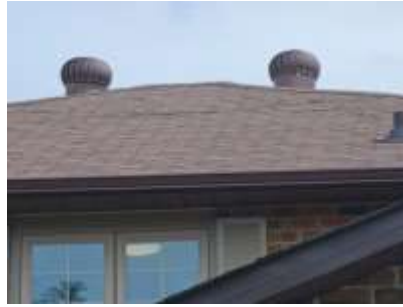
Pic. 2: Roof covering – appears one shingle tab is torn
