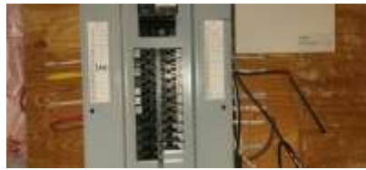
Pic. 32: 200-amp breaker panel
