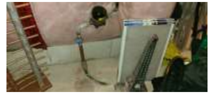
Pic. 33: Water main
