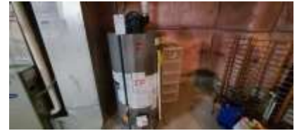
Pic. 30: Rental hot water tank 2022
