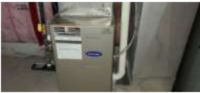
Pic. 31: Gas furnace 2010
