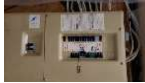
Pic. 35: 100 amp breaker panel
