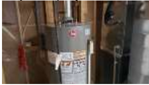
Pic. 33: Rental hot water tank
