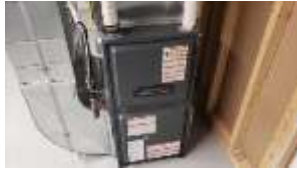
Pic. 34: Gas furnace 2015
