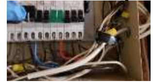
Pic. 36: One breaker double tapped
