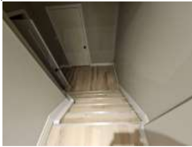
Pic. 32: Handrailing advised for stairwell
