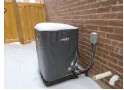
Pic. 3: AC unit
