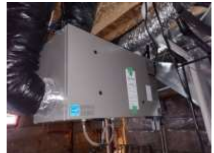
Pic. 30: HRV system
