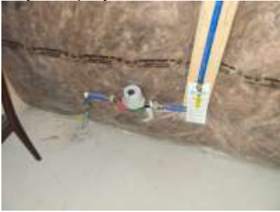
Pic. 31: Water main
