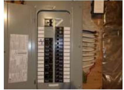
Pic. 33: 100 amp breaker panel
