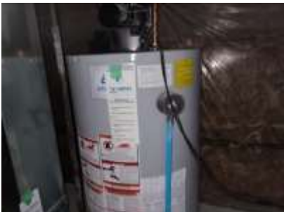
Pic. 28: Rental hot water tank
