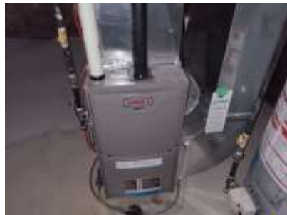
Pic. 29: Gas furnace
