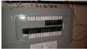
Pic. 10: 100 amp breaker panel
