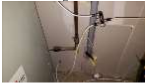
Pic. 9: Water main
