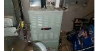
Pic. 8: Gas furnace 2012
