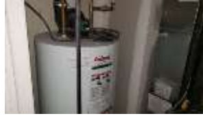
Pic. 7: Rental hot water tank
