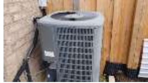
Pic. 6: AC unit 2007
