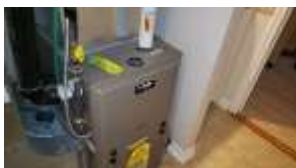
Pic. 29: Gas furnace 2013
