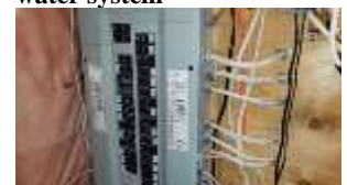
Pic. 32: 100 amp breaker panel
