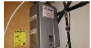
Pic. 28: Rental tankless hot water system
