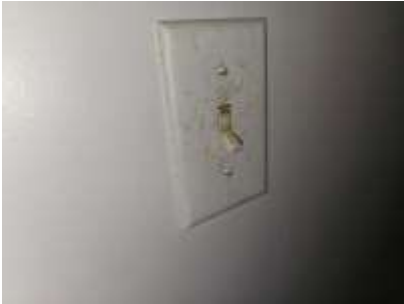
Pic. 37: Light switch for basement stairwell defective
