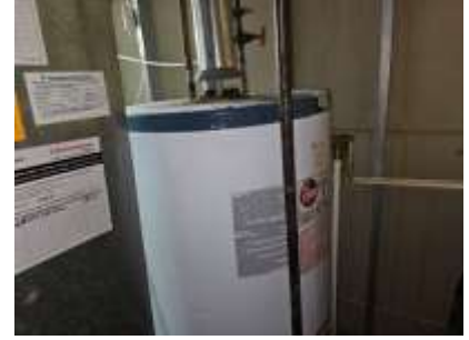
Pic. 33: Water heater 2005
