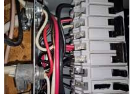
Pic. 36: Double tapped breaker
