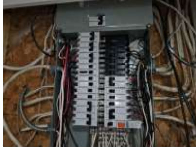
Pic. 35: 100 amp breaker panel
