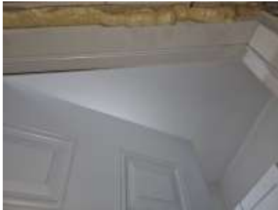
Pic. 7: Auto closer advised for garage entry door
