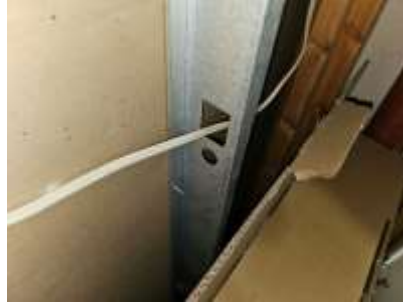
Pic. 32: Wiring installing incorrectly in basement
