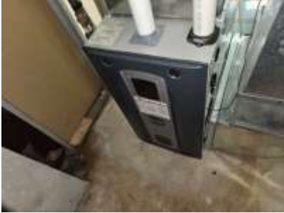
Pic. 34: Gas furnace 2022
