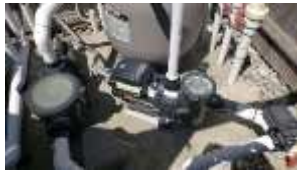
Pic. 14: Pool pump
