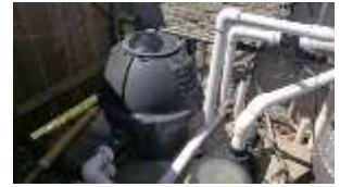
Pic. 12: Pool heater
