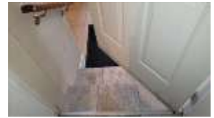
Pic. 16: Garage entry door wrong swing
