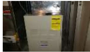
Pic. 47: Gas furnace 2001
