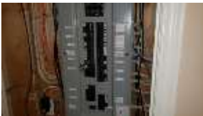
Pic. 49: 200 amp breaker panel
