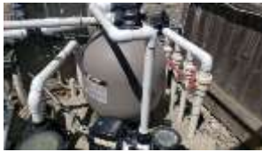
Pic. 13: Pool filter
