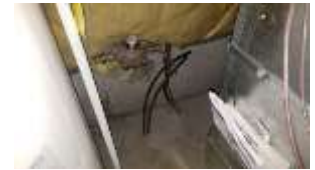
Pic. 48: Water main
