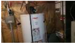
Pic. 46: Rental hot water tank
