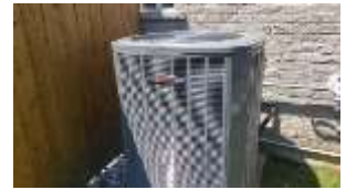
Pic. 4: AC unit 2016
