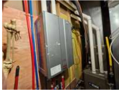
Pic. 20: Tankless hot water
