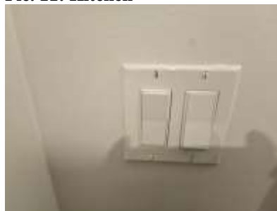
Pic. 14: Exhaust fan switch faulty and should be replaced
