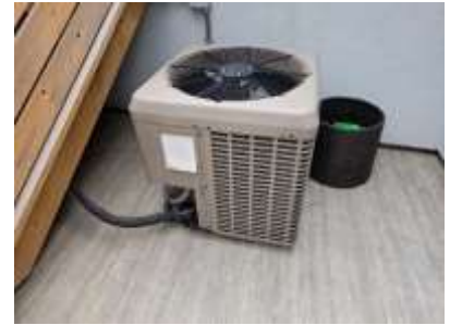
Pic. 6: AC unit
