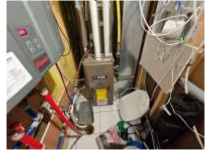
Pic. 21: Gas furnace
