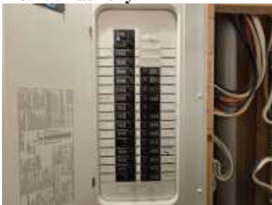
Pic. 22: 100 amp breaker panel
