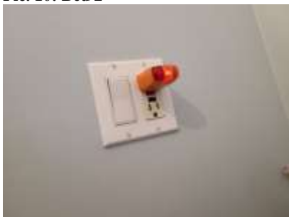
Pic. 13: Open ground outlet in bathroom and most of the main floor
