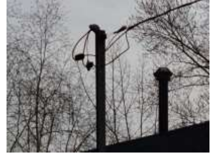
Pic. 3: Service drop
