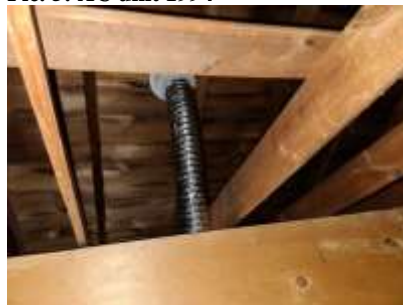
Pic. 8: Vent pipe in attic should be insulated
