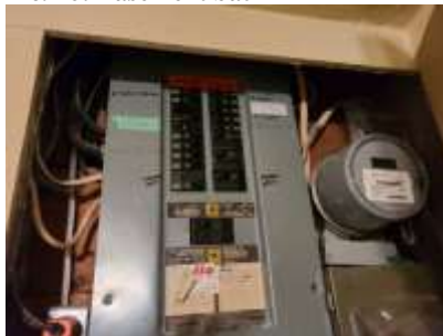
Pic. 29: 100 amp breaker panel
