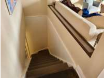
Pic. 19: Handrailing advised for basement stairwell
