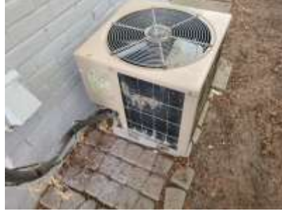
Pic. 5: AC unit 1994
