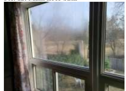
Pic. 15: Blown window seal
