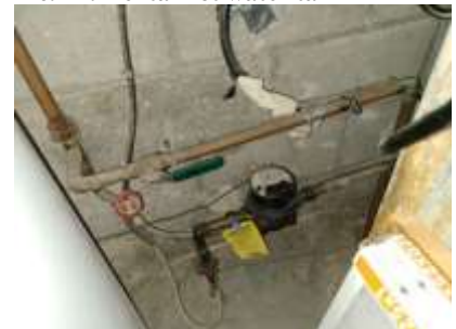
Pic. 30: Water main
