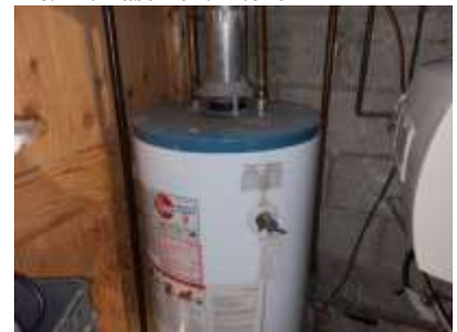
Pic. 27: Rental hot water tank
