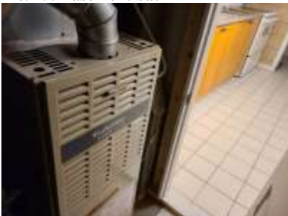
Pic. 28: Gas furnace 2001
