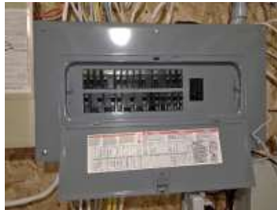
Pic. 35: 100 amp main electrical panel
