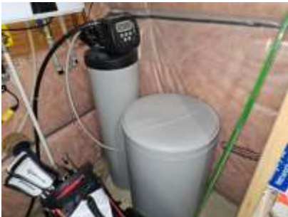
Pic. 34: Water softener
