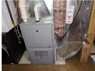
Pic. 32: Gas furnace 2010
