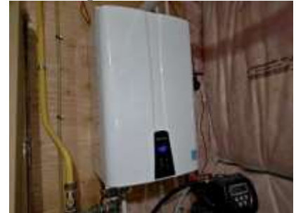
Pic. 33: Tankless hot water system 2014
