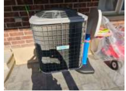
Pic. 6: AC unit 2010
