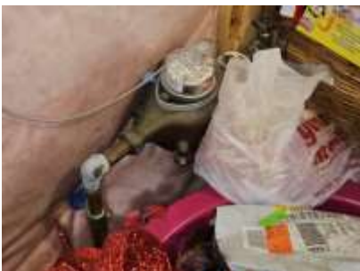
Pic. 37: Water main
