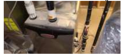
Pic. 24: Gas furnace 2017
