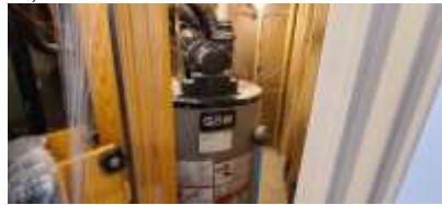
Pic. 23: Rental hot water tank
