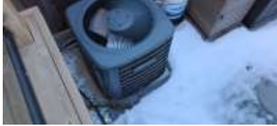
Pic. 4: AC unit
