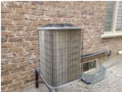
Pic. 4: AC unit 2015
