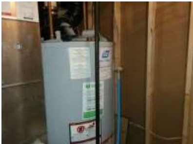
Pic. 37: Rental hot water tank
