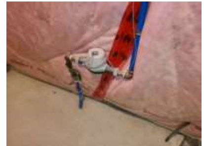
Pic. 39: Water main
