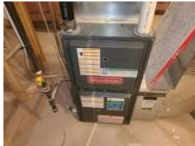
Pic. 38: Gas furnace 2015
